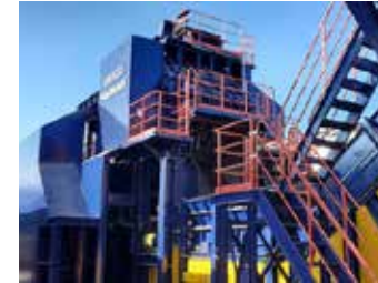
ECONECOL Inc. Matsumoto Plant Pre-Shredder
